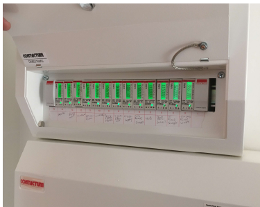
Every electrical circuit in the house is monitored.
