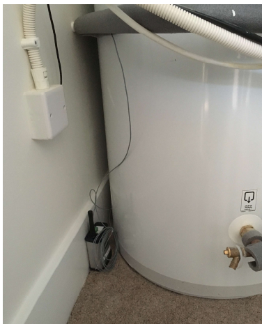
Monitoring the hot water system
